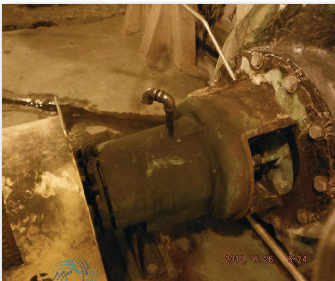
Figure 4: "Gooseneck" vents such as these should be avoided
